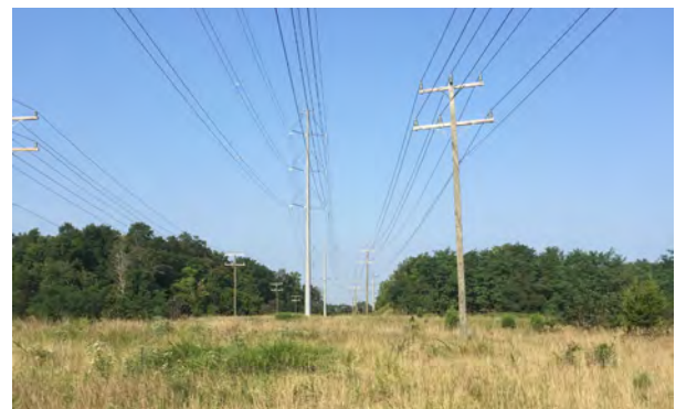
Figure 7. Overhead Power Lines Crossing Prentice Drive
