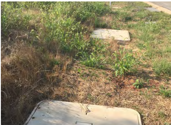
Figure 9. Underground Communication Lines
