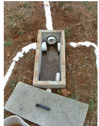
Example of a Distribution box
